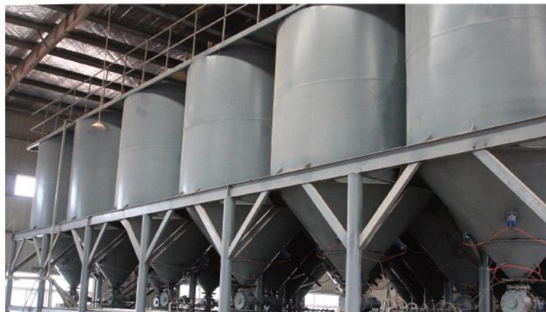
储量达12000吨的成品泥料储存系统 Reserves of 12000 tons of finished clay materials storage system
